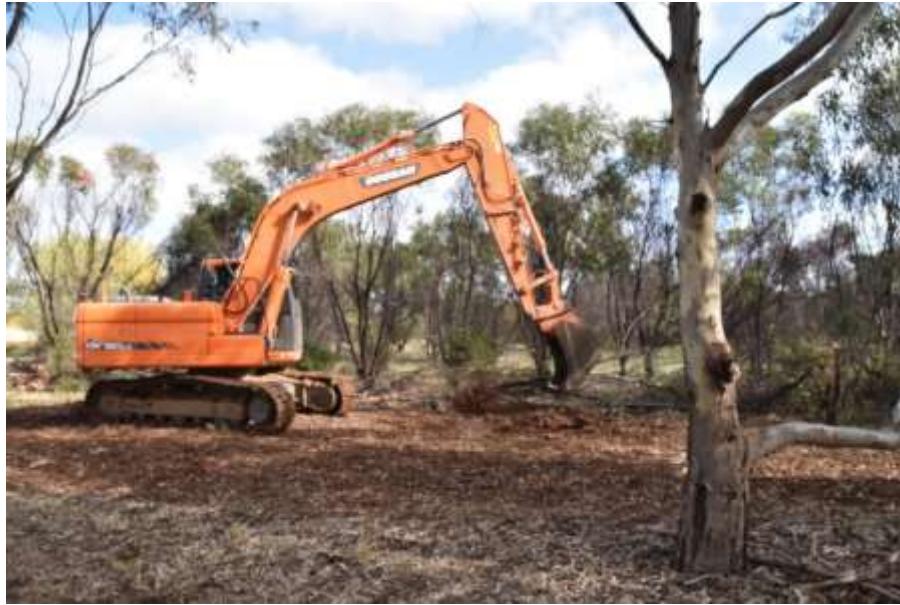
Figure 12. An excavator removes Acacia pycnantha plants which were unproductive. Photo by S Logie.
