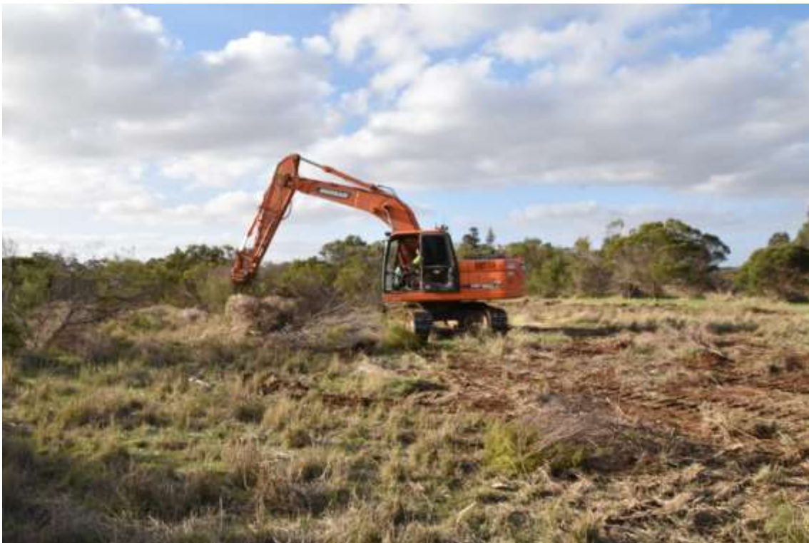
Figure 2: SPA Renovation: An excavator removes shrubs at a Berrigan SPA. Photo S Logie
